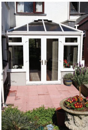
Double Edwardian with box gutter to three sides, plus parapit wall with lead valley to back side.
